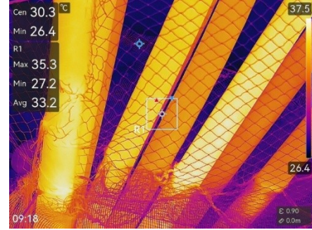
Fig 6 Infrared Thermal Capture
