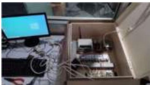
Figure 7. Automatic Irrigation Control Panel
