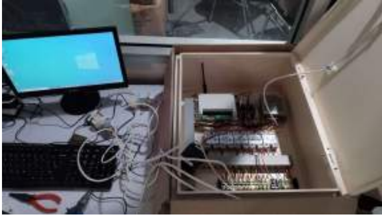
Gambar 10. Panel kontrol automatic irrigation
