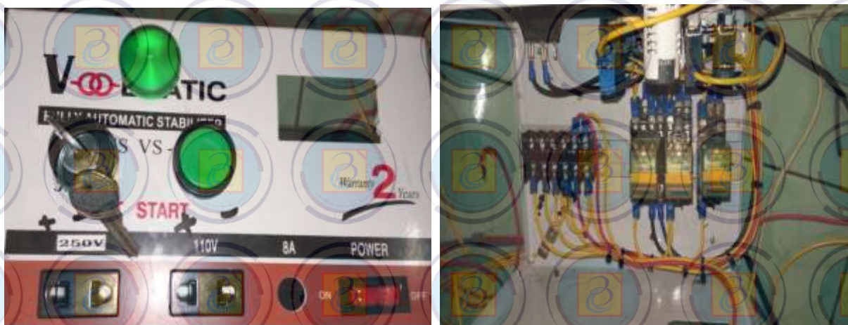
Gambar 5: Hasil Perancangan Box Panel Unit Genset
