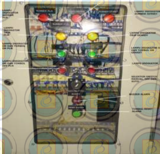
Gambar 3: Tampak luar Panel ATS/AMF
